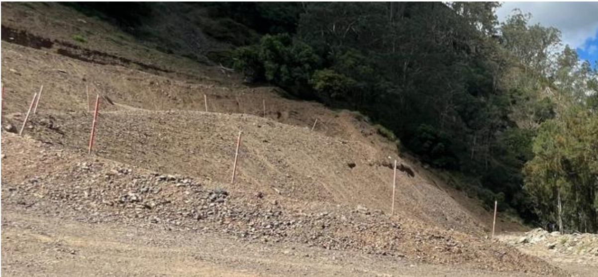
Figure 41: The Bakers Creek Waste Dump lower area, very poor vegetation take-up on steeper slopes - March 2023
