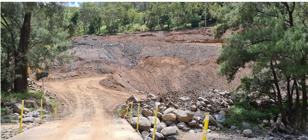
Figure 39: The Bakers Creek Waste Dump at the final stage, with the permanent road in place - January 2022.
