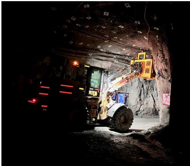
Figure 3 UG Electrical Upgrades for more powerful Jumbo mining machines
