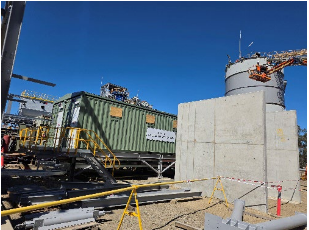
Figure 1 New Electrical Switchroom, concrete blast bunker for upgraded transformer and raised ore bin at rear
